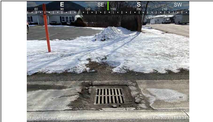
17.) View of stormwater catch basin along NY-54. Catch basin appears to discharge to the east. See photo 19 for concrete outlet.
