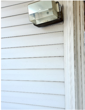
FIGURE 28: EXTERIOR WALL PACKS (EACH FIXTURE SHALL BE REPLACED IN ITS ENTIRETY)
