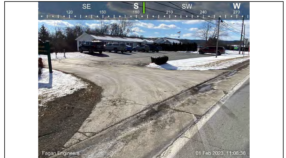
4.) Paved entrance has cracks in several locations.
