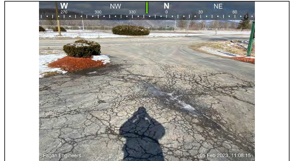
2.) Cracks spreading near the entrance. Area is beginning to form a pothole.
