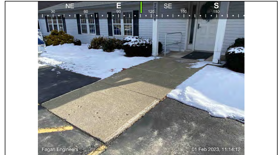
10.) Concrete sidewalk to the front of the building. Wheelchair accessible ramp constructed (see photo 11).
