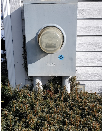
FIGURE 17: EXISTING MAIN METER
