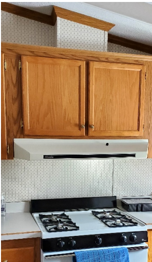
FIGURE 16: EXISTING RANGE EXHAUST FAN
