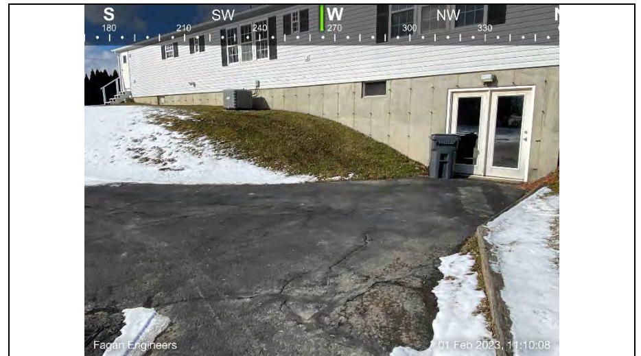
8.) View of pavement to the rear of the building. Pavement cracks can be observed. Cracks appear to have been repaired in the past but have continued to spread.
