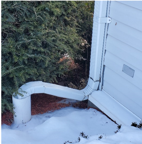
FIGURE 8 EXISTING GUTTER ISSUE
