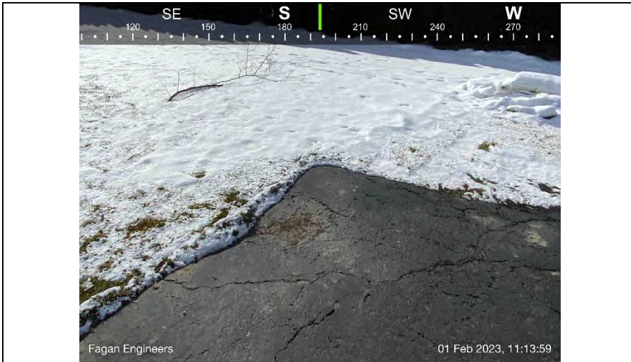
13.) View of asphalt sinking at the corner of the pavement.
