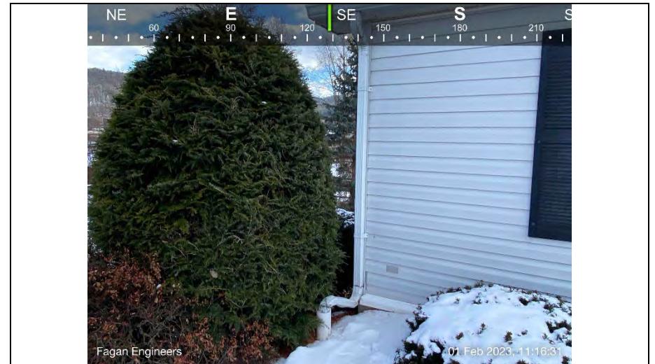
16.) View of roof leader extending into the ground off the northwestern corner of the building.
