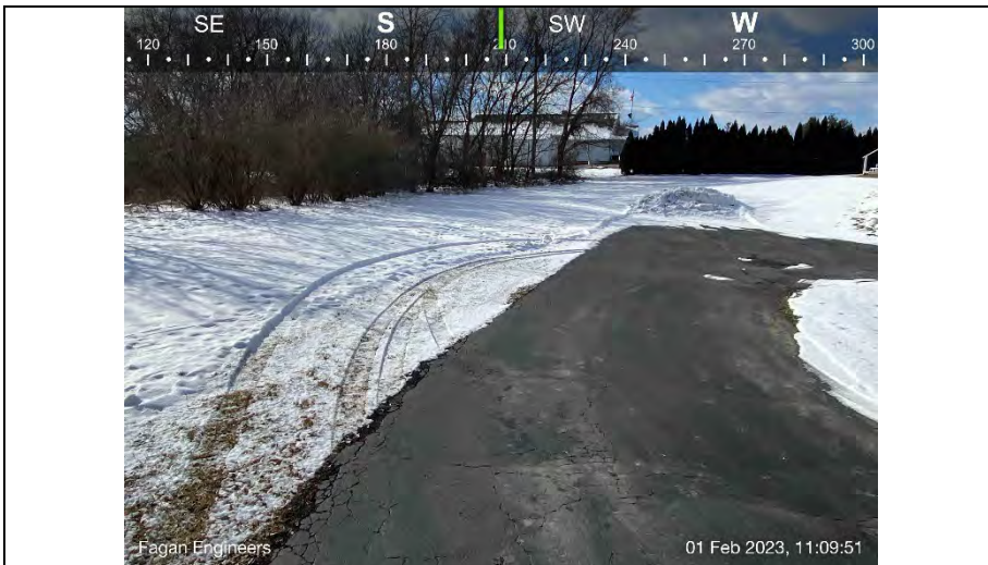
7.) View of the pavement to the rear of the property. Vehicles accessing the rear of the property appear to drive on the lawn due to pavement restrictions.
