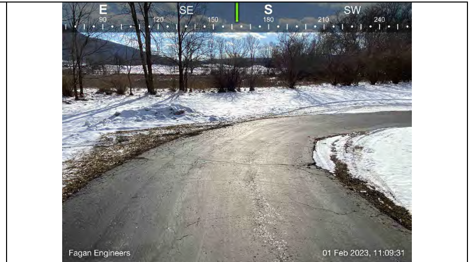
6.) View of the radius to the rear of the building. Rutting can be seen on either side of the asphalt. Small cracks were observed throughout.
