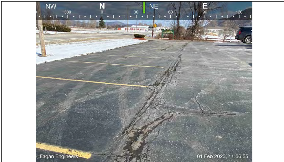
1.) Pavement cracking along the seam. Cracks are becoming too large to resurface/repair.
