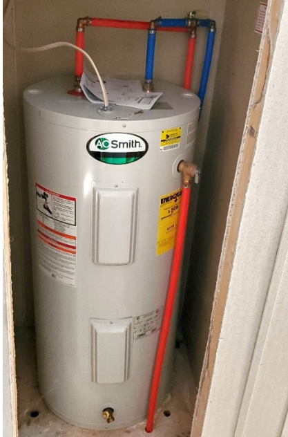
FIGURE 5: EXISTING WATER HEATER
