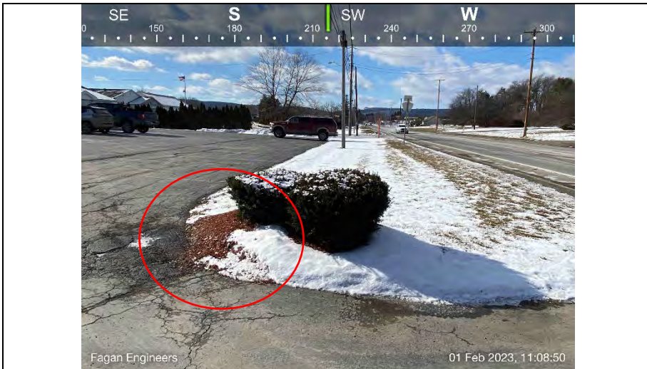
3.) Landscaping/bush on the southern radius of the entrance. Landscaping appears to be consistently driven over.
