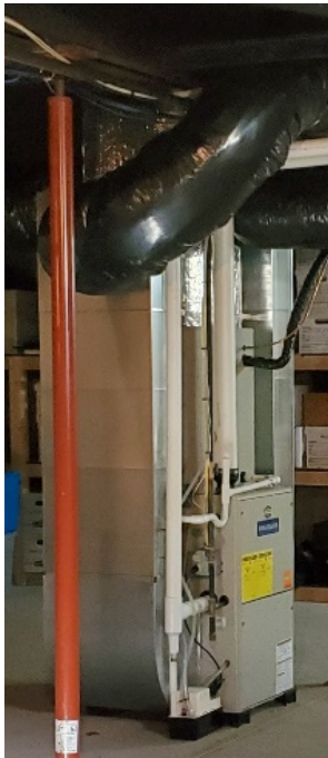
FIGURE 14: EXISTING FURNACE AND COOLING COIL
