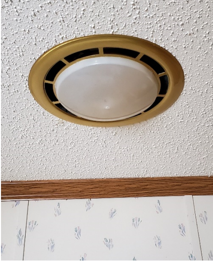
FIGURE 15: EXISTING BATHROOM EXHAUST FAN
