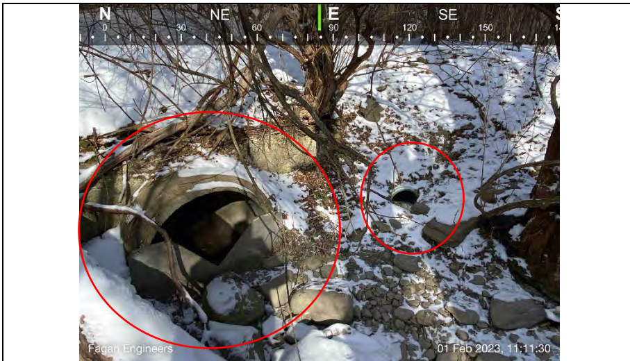
19.) View of stormwater discharge pipes from the catch basin on NY-54 (left) and the catch basin to the rear of the target property (right)
