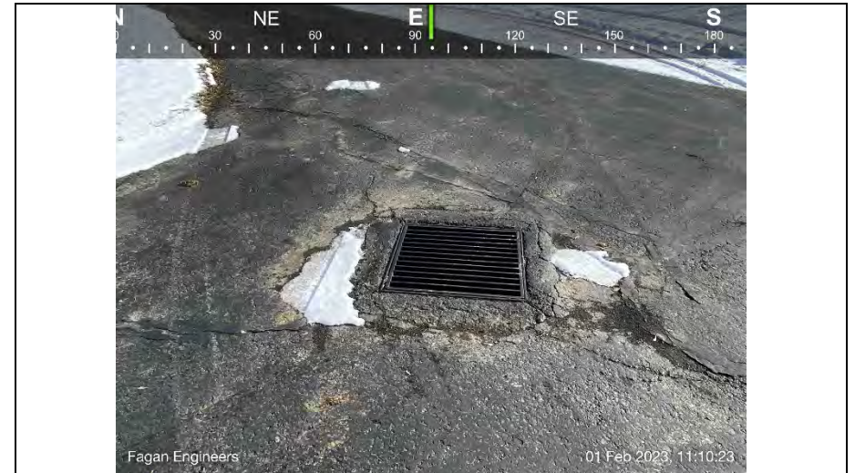
18.) View of the catch basin to the rear of the structure. Catch basin was estimated to be halfway full of water at the time of the inspection. Asphalt/concrete surrounding the structure requires repair.
