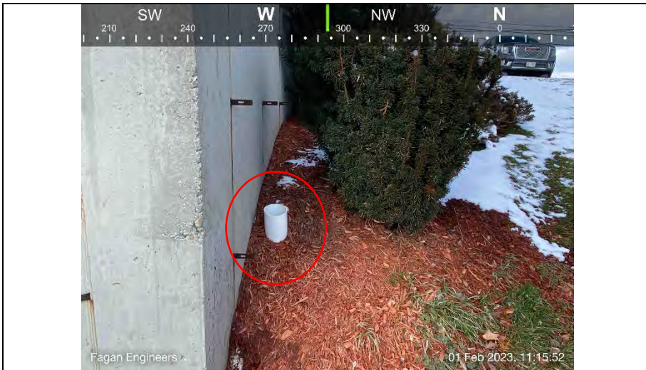
15.) View of what appears to be a roof leader pipe just off the northeastern corner of the building.
