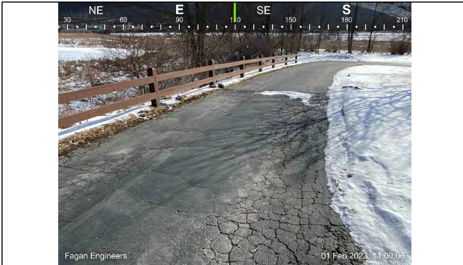
5.) View of the asphalt access road leading to the rear of the building. Pavement can be seen breaking down from vehicle traffic.
